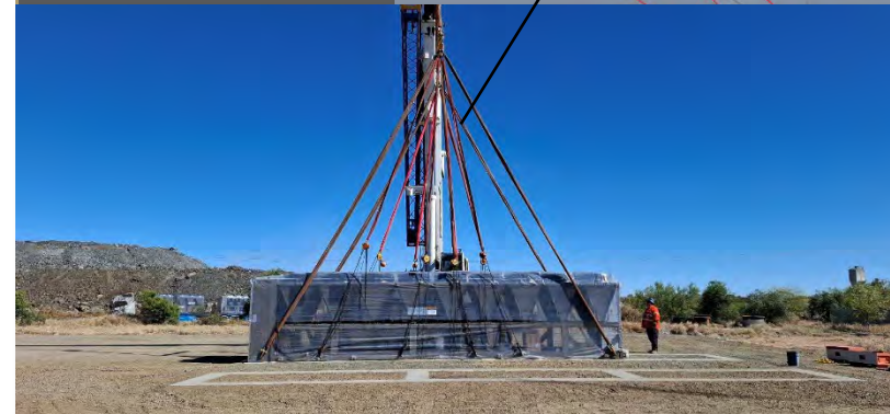
Bulk Air Cooler first delivery
